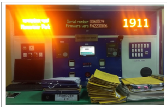
Figure 2. The PA system test bench at the Electronics Lab, Delhi metro. Source: Author's personal collection.
